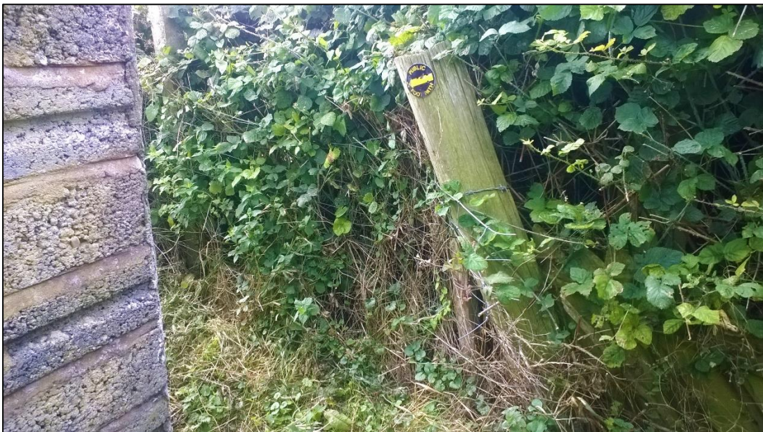
Illustration 5: Remove rotten corner post and other timber posts and re-use existing concrete posts.
